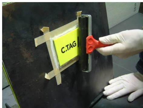
12. A roller can be also used to ensure 100% contact between C.TAG/® marker and substrate.
